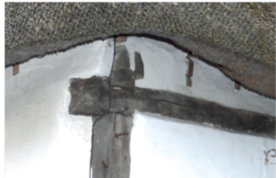
Exposed timber in mud and stud wall © Naomi Field
