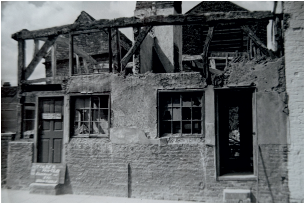
Rare example of a two-storey building during demolition. This example from Louth illustrates many of the terms in the glossary
